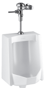
Existing urinal and flush valve
